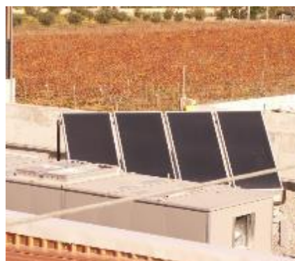
Figure 2: Winery with a ST system in the roof.
