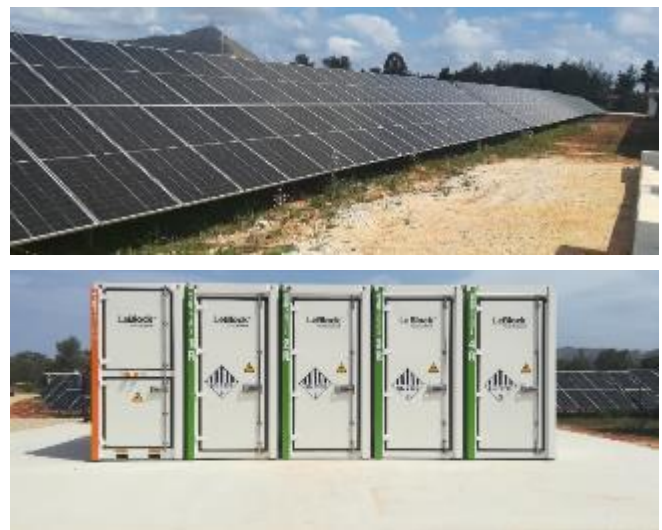
Figure 10: The Lighthouse Project in Chania Airport: PV panels and BESS
